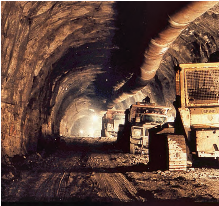
Construction of the cooling water intake tunnel at Darlington in the Cobourg Formation provided evidence that the formation can sustain a stable, dry opening
