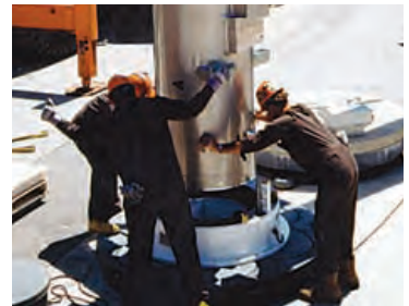
Intermediate level nuclear waste is inserted into an in-ground storage container at the WWMF
